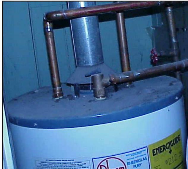
Stand-alone gas water heaters are the most likely appliance to suffer draft reversal
