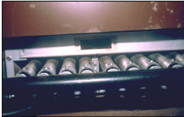
Atmospheric natural gas burners on a large boiler
