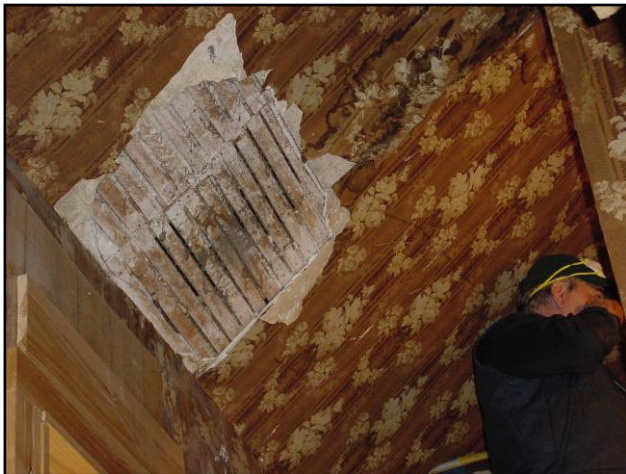
A significant air bypass in a closet up into a sloped ceiling through plaster and lath
