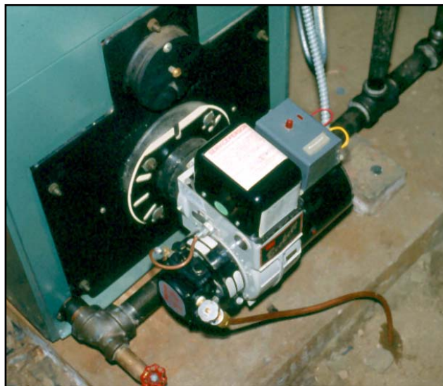
Flame retention head oil burner on a wet base boiler
