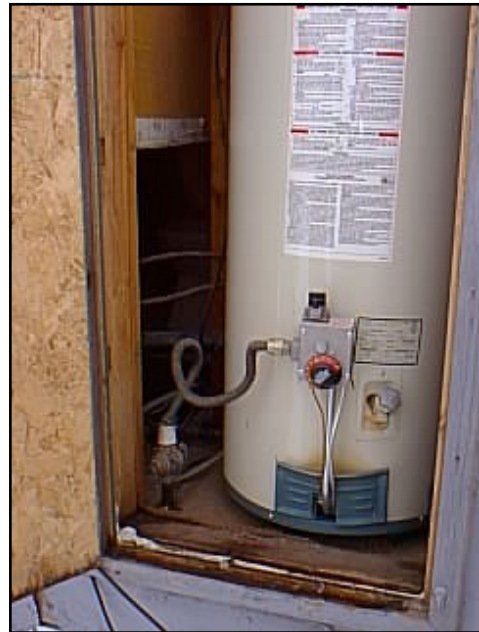
Mobile home water heater closet with gas-fired water heater
