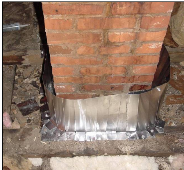
Chimneys must be blocked to keep cellulose at least two inches away from the masonry
