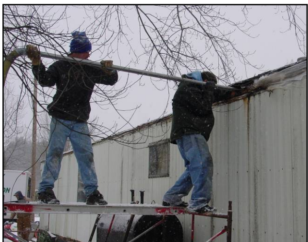
Blowing a mobile home roof from the edge
