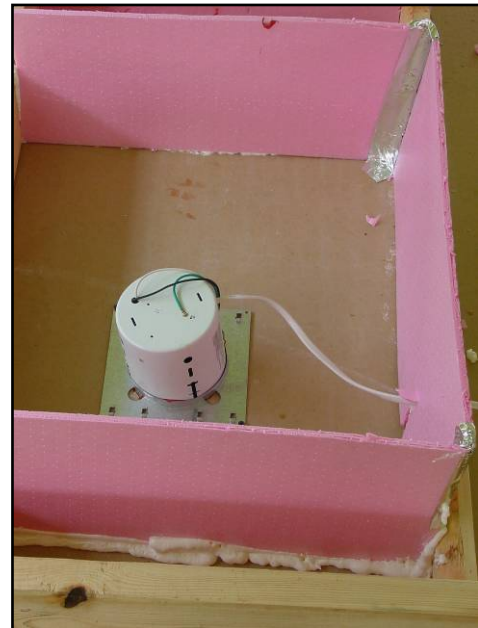
This blocking allows too much space around this recessed light; insulation must be kept just three inches away
