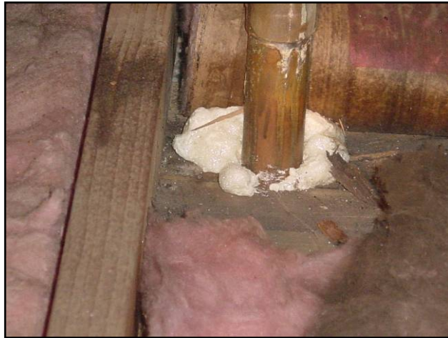
Plumbing stack sealed with foam
