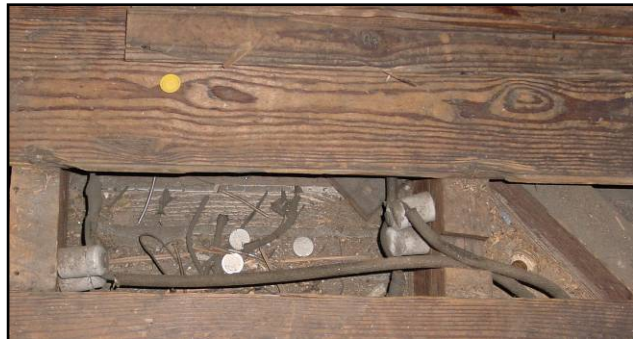
Even if there is attic flooring, knob-and-tube wiring and attic bypasses must be found and treated before insulation is added
