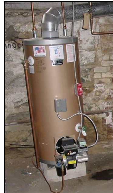
Oil-fired water heaters are not common
